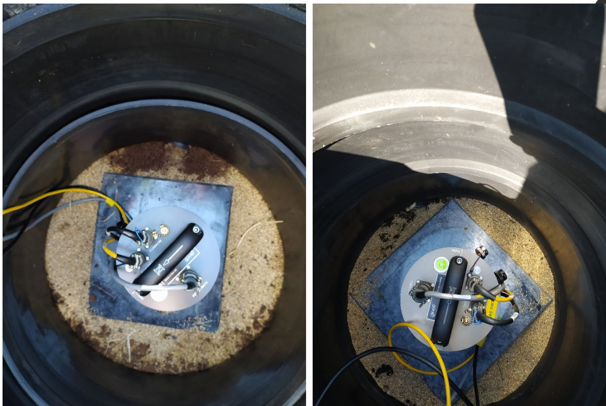
Figure 17 - Installation of the sensors at two measurement locations. Sensor resting on the slab prior to being covered by insulation.
