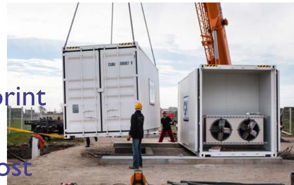
Installation of Pellworm containerised battery
